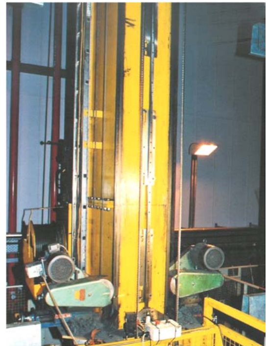
The 22 Metre High Stacker Mast
